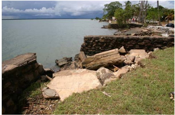
Fig. 6 Damage to the sea wall caused by a stormtides on Saibai in 2006 (photo credit: Donna Green)
